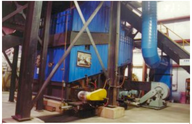
Picture 1 CHP Facility, Taylor Lumber, NS Courtesy of KMW Energy Inc.
